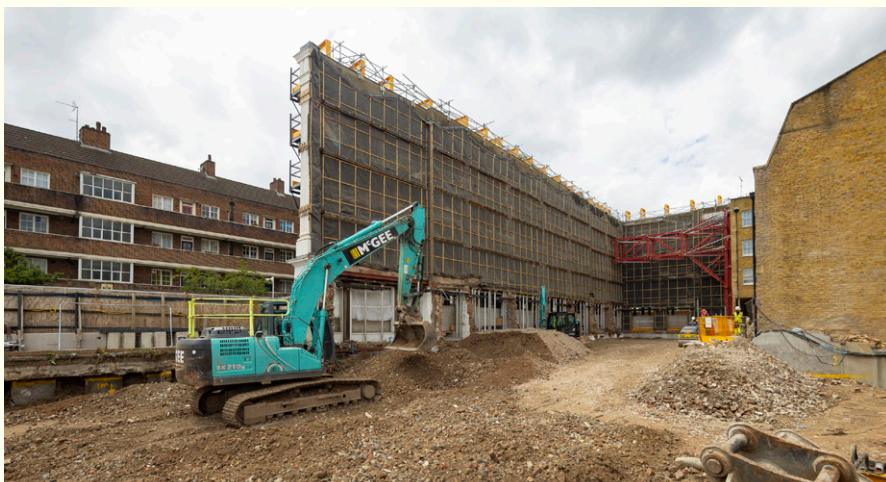
BLOCK 9: View behind the facade where the new 'Block 9' building will be constructed.
