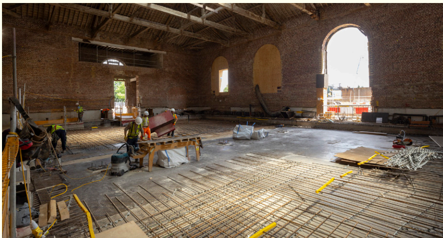
NEW FLOOR SLAB FOR THE RIDING SCHOOL: View of the extensive works going on inside the Riding School to pour the new concrete floor.
