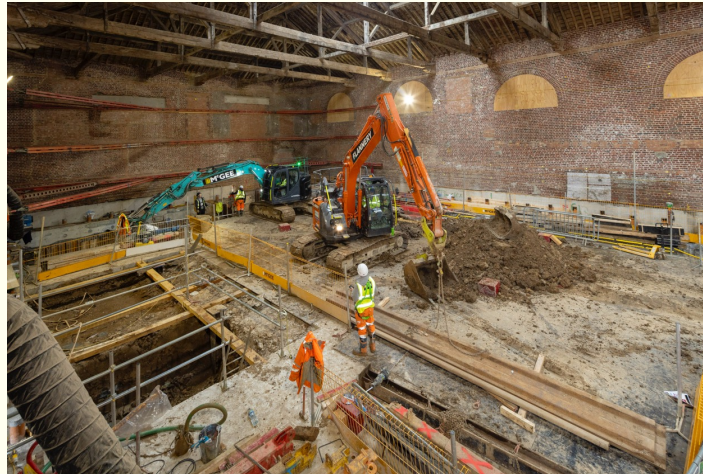
RIDING SCHOOL: Shaft excavation, underpinning, and basement works are taking place within the Riding School.
